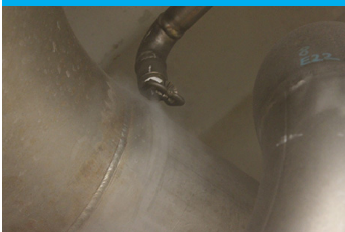
DAMAGED DELUGE NOZZLE
