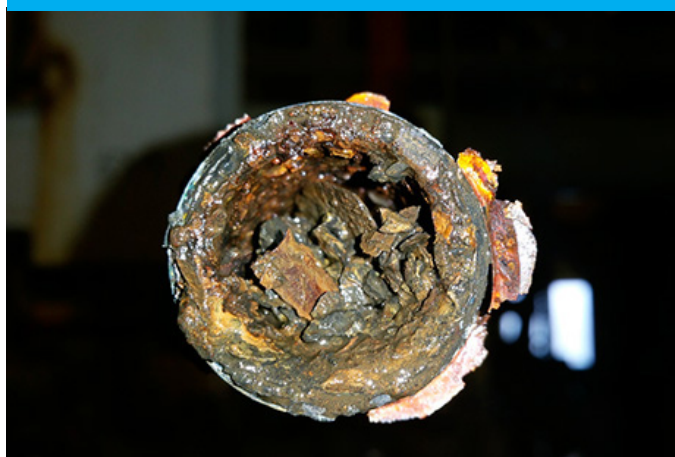
FULL DELUGE PIPEWORK BLOCKAGE
