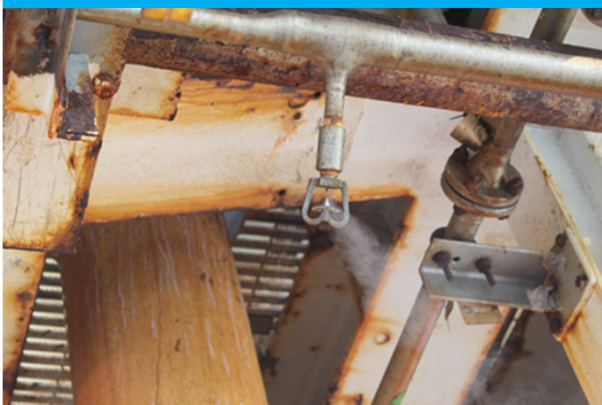
PARTIAL DELUGE NOZZLE BLOCKAGE
